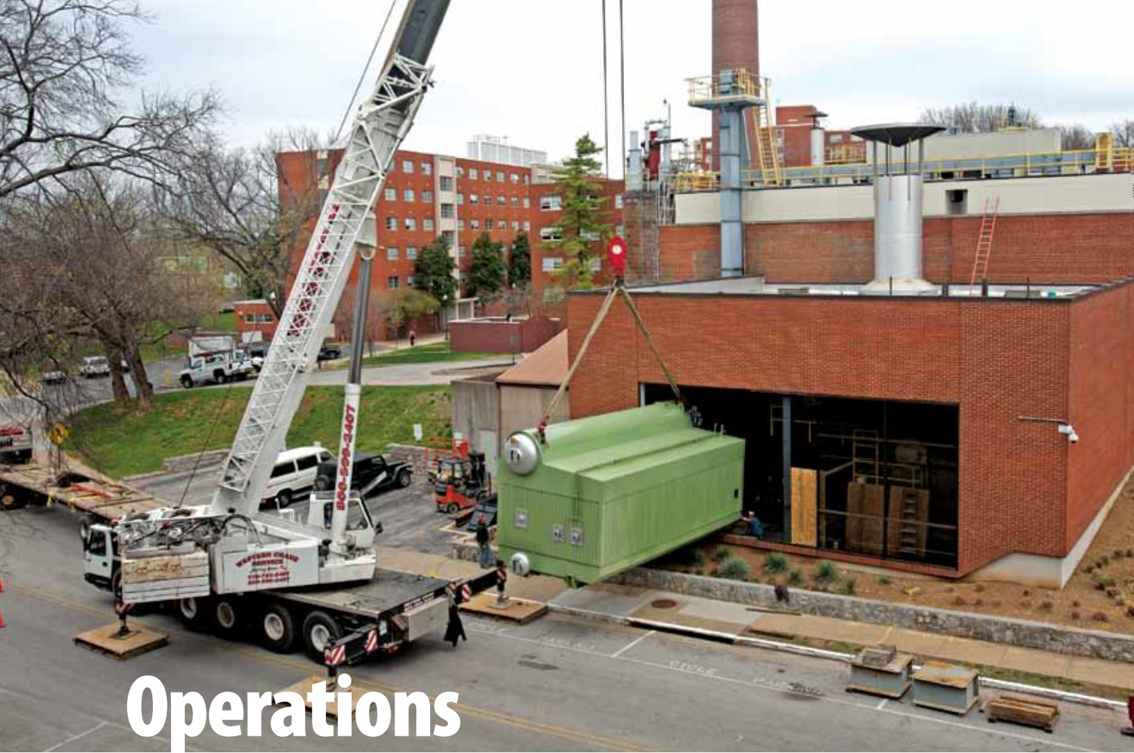
◀ Installation of natural gas boiler #2 in spring 2011. This boiler completed the Central Heating Plant upgrade, allowing for complete heating with natural gas. The project was funded by utility budget savings resultant from conservation and efficiency programs.
