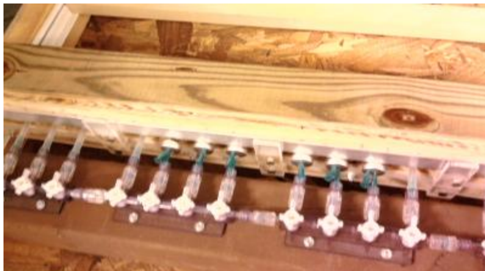
Figure 2.10. Nitrogen gas manifold.
