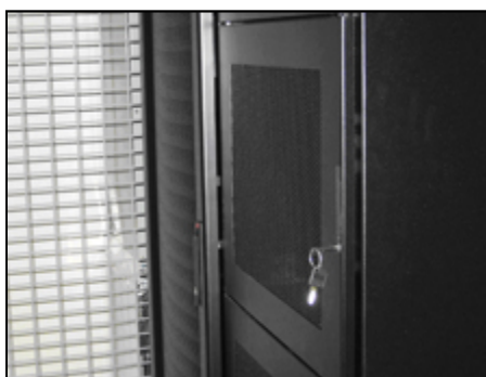
Figure 3-1. Rack space rented from Bowling Green Municipal Utilities. (Source: BGMU 2010).
