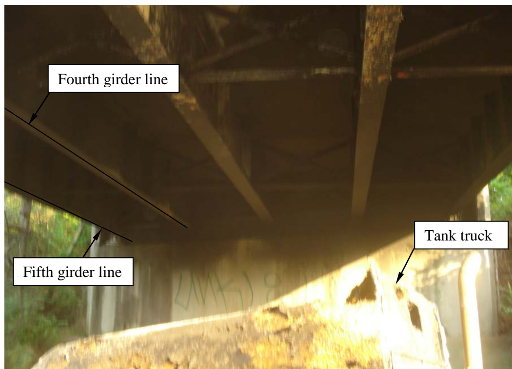
Figure 57. Position of tank truck beneath Lime Kiln Lane overpass (facing toward the east end abutment).
