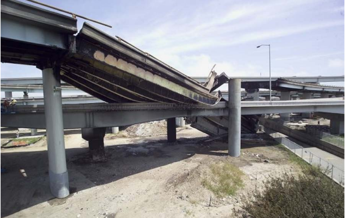
Figure 23. Damage caused by MacArthur Maze fire (© 2007 California Department of Transportation).
