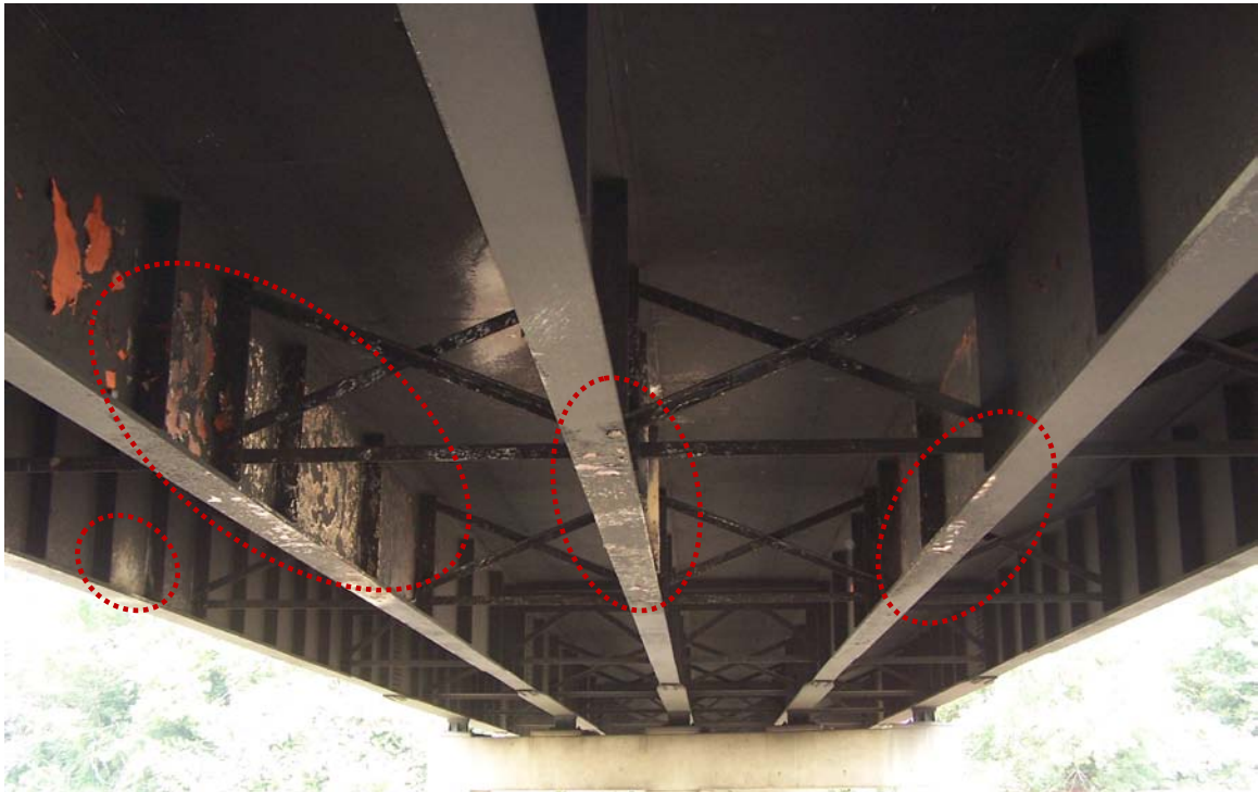
Figure 55. Girder damage caused by the Lime Kiln Lane overpass tank truck fire (west view from east-end abutment).
