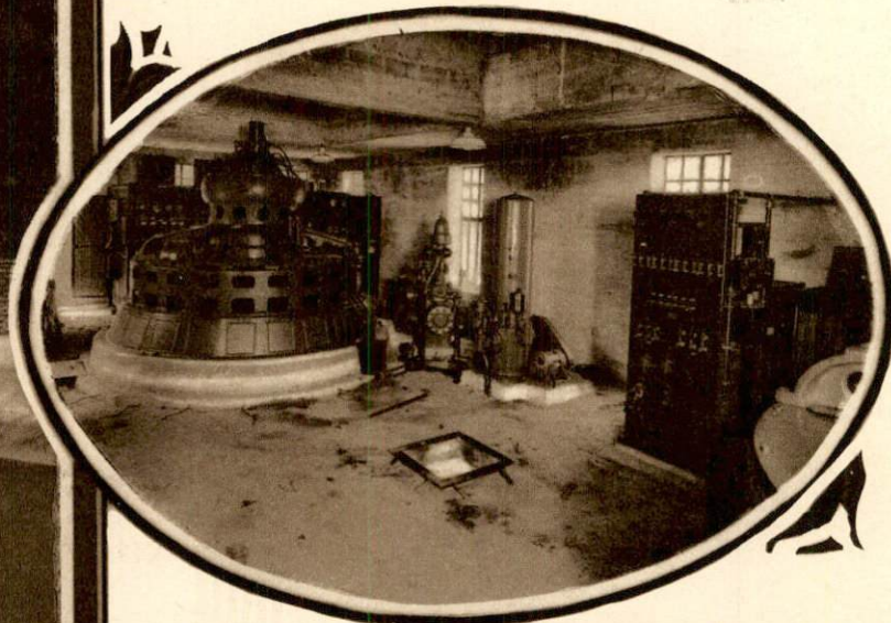
(Above): Interior of hydro-electric plant on Lock No. 7. This station is connected with the big plant at Dix Dam. —Lafayette Studio.
