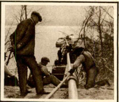
Laying pipe line under Ohio River to carry natural gas from Western Kentucky to northern states.
