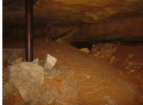
Figure 7. Micropile under the Skydome: A micropile breaching the northern cave passage that was installed to support the Skydome structure before the remediation of the sinkhole was initiated.
