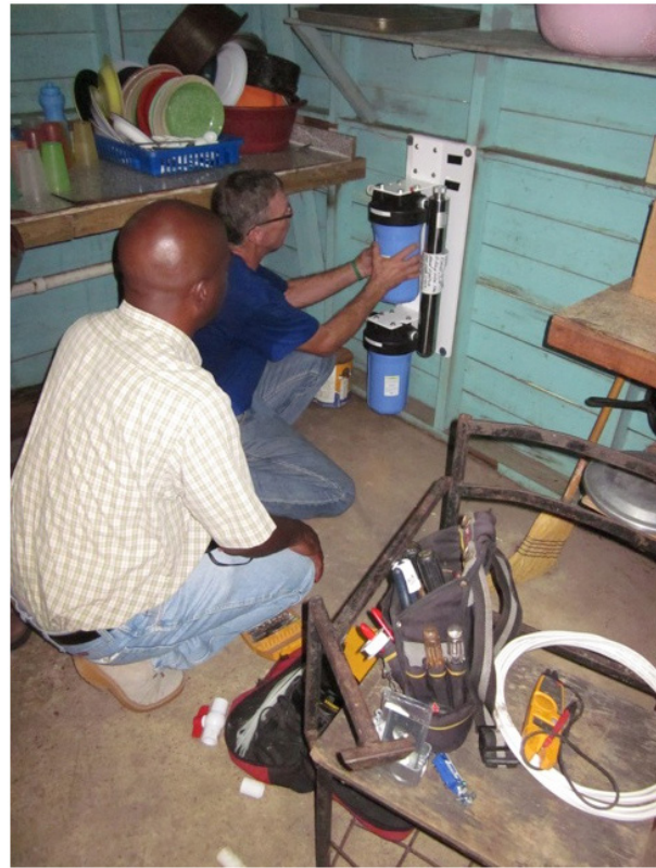
Figure 7. AJ Strenecky of the Goshen Rotary and Mr. Anthony Flowers of the Ministry of Health inspecting the newly installed UV water purification system (photo by Jason Polk).
