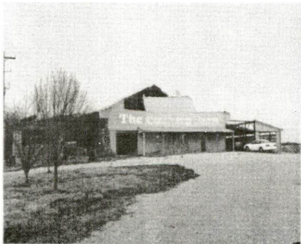
South facade of barn. A third of the roof structure was blown off, as well as extensive damage to both sheds.
