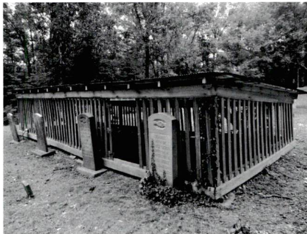
The grave house of Elias (1849-1919) and Jennie (1844-1935) Wood. This structure is crowned with an unusual shed roof and covers four graves. The opening which once featured a gate allowed access for family members to go in and clean the grave or leave flowers of mementos. This grave house is located in the New Hebron Baptist Church Cemetery in southern Muhlenberg County.
