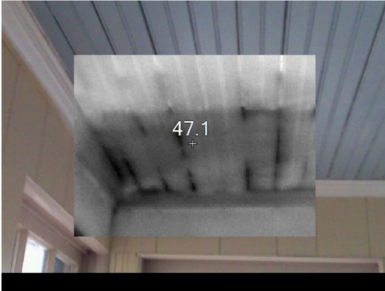
Figure A.12. Warm Air Escape through Sunroom Ceiling. Source: Robert E. Choate. (2013). "Energy Audit Baseline Study".
