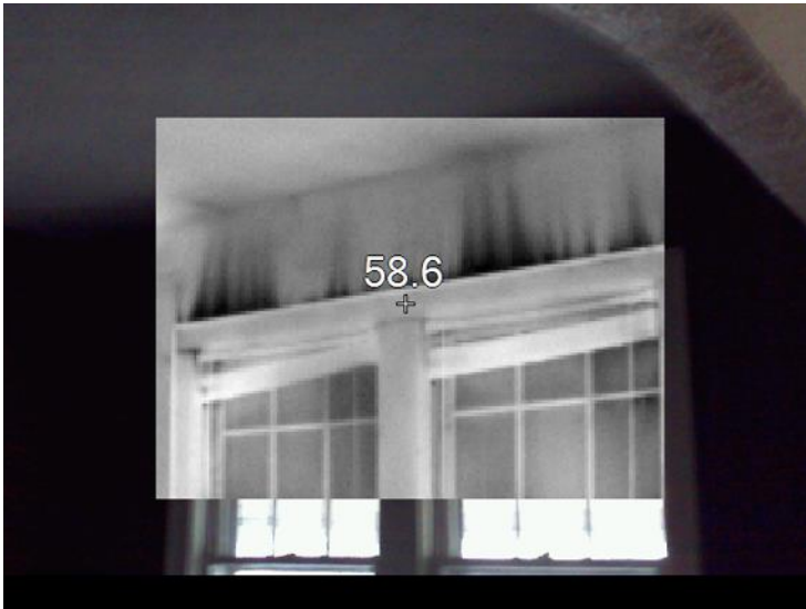
Figure A.3. Cold Air Infiltration around Foyer Windows. Source: Robert E. Choate. (2013). “Energy Audit Baseline Study”.
