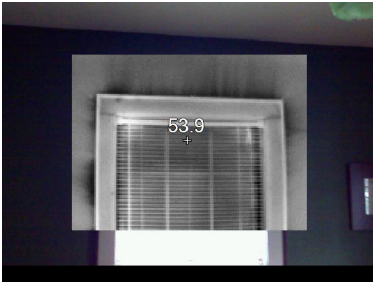
Figure A.1. Cold Air Infiltration around Big Red Bike Office Window. Source: Robert E. Choate. (2013). “Energy Audit Baseline Study”.
