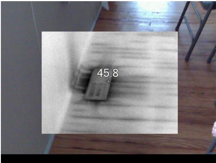
Figure A.11. Cold Air Infiltration around Sunroom Ventilation Installation. Source: Robert E. Choate. (2013). "Energy Audit Baseline Study".
