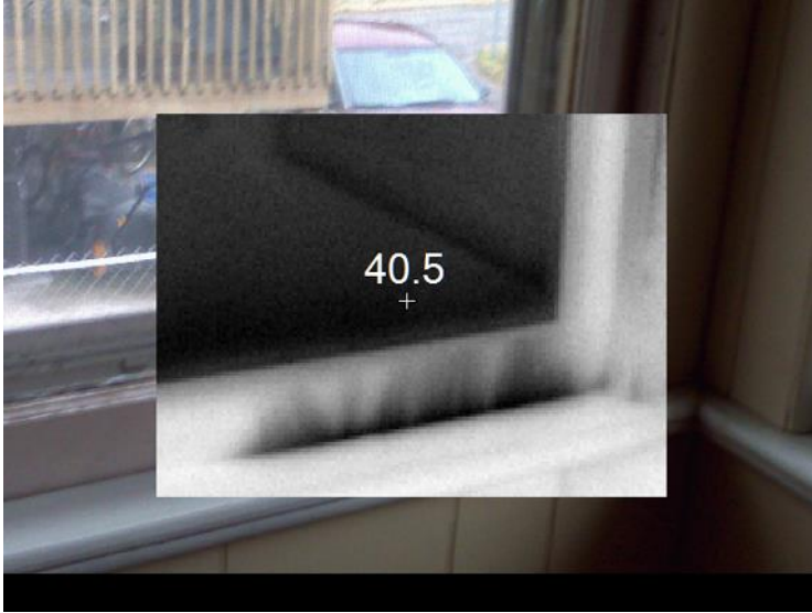
Figure A.4. Cold Air Infiltration and Warm Air Escape around Sunroom Window. Source: Robert E. Choate. (2013). “Energy Audit Baseline Study”.
