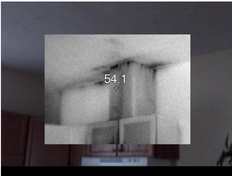
Figure A.9. Warm Air Escape around Kitchen Ventilation Installation. Source: Robert E. Choate. (2013). “Energy Audit Baseline Study”.
