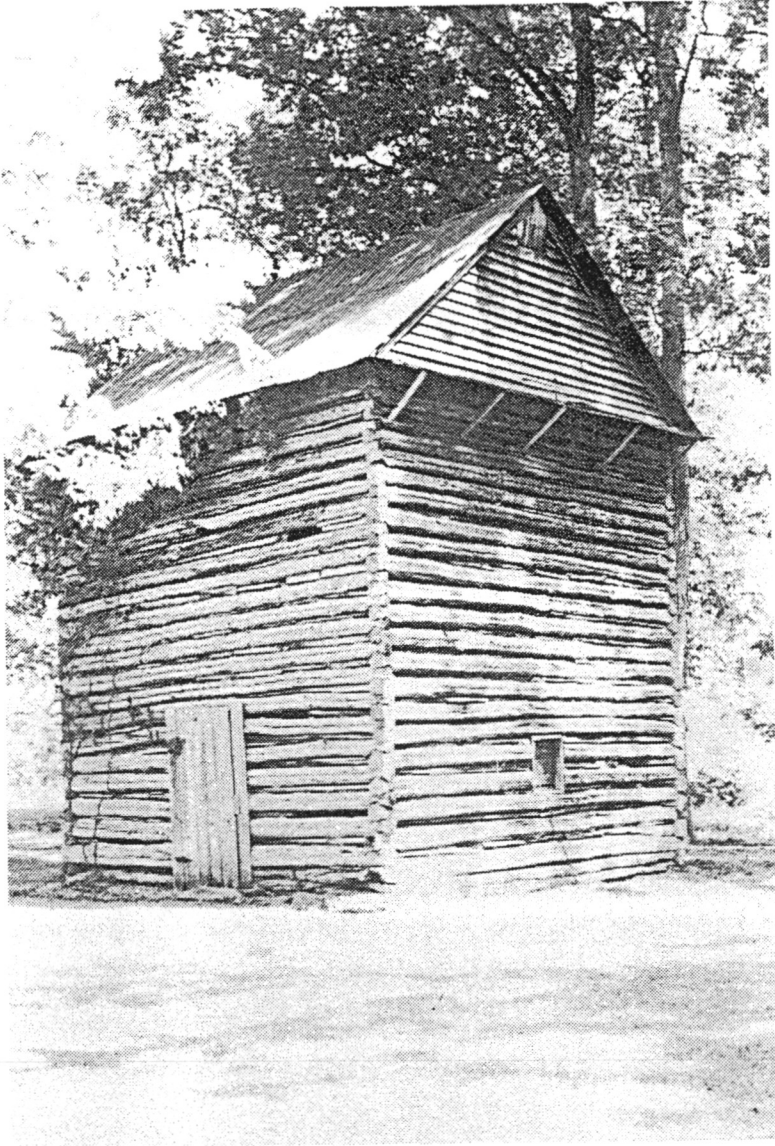
This barn, also at the Tidwell site, is identical to the previously described structure. It is believed to be in excess of ninety years old.
