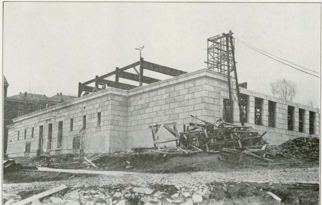
The new $200,000 Library is being rapidly constructed. It occupies the site of the old Home Economics Building.
